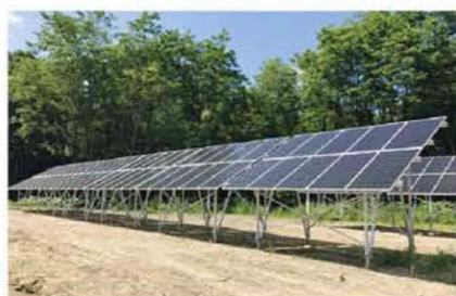
200KW in Qatar
